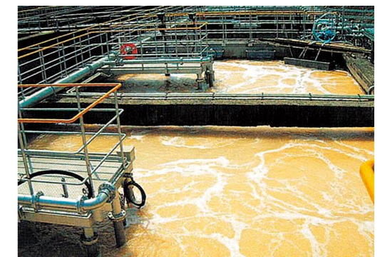
Facilities applying the new waste water treatment system in the Kuraray Saijo Plant
