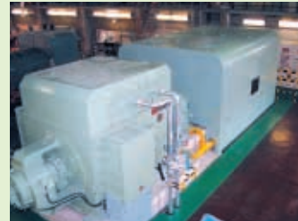
Condensing turbine generator at the Niigata Plant
