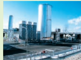
A natural gas storage facility at the Okayama Plant
