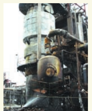
The vicinity of a reactor damaged in the explosion
