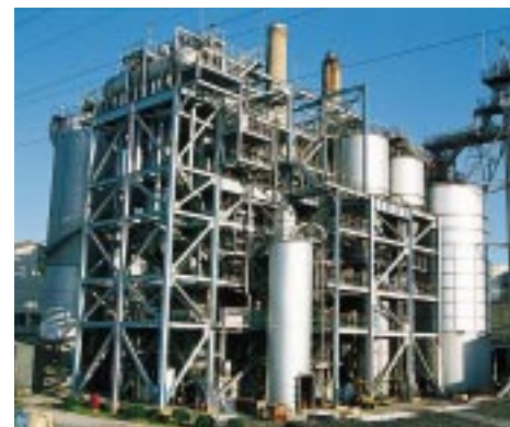
Fluidized bed boiler at the Tamashima Plant
